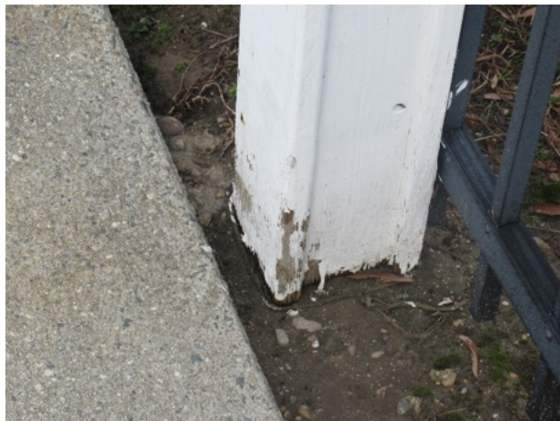
Pole finish deterioration
