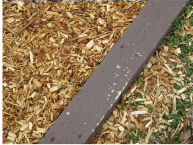
Wood deterioration at pool house
