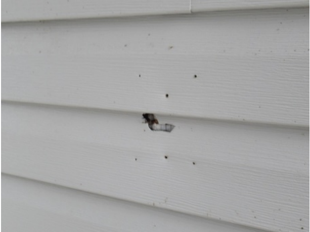
Pool house siding damage
