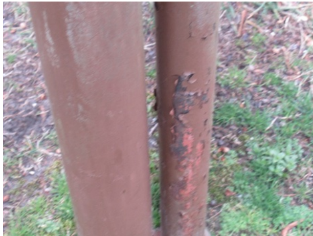
Rust and finish deterioration
