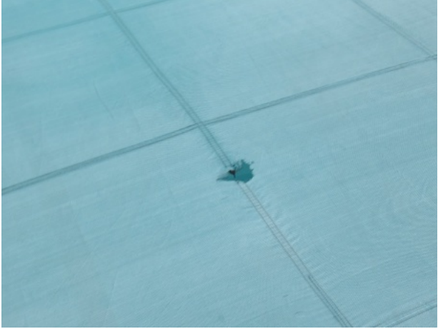
Main pool cover hole
