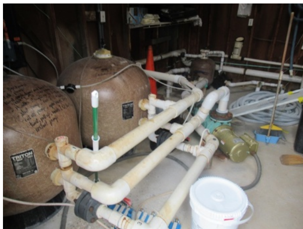
Pool equipment overview
