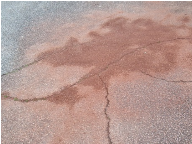
Cracks and water seepage
