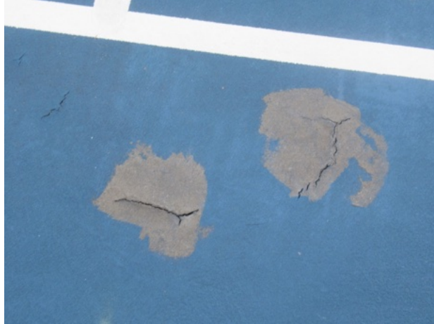
Cracks and paint deterioration
